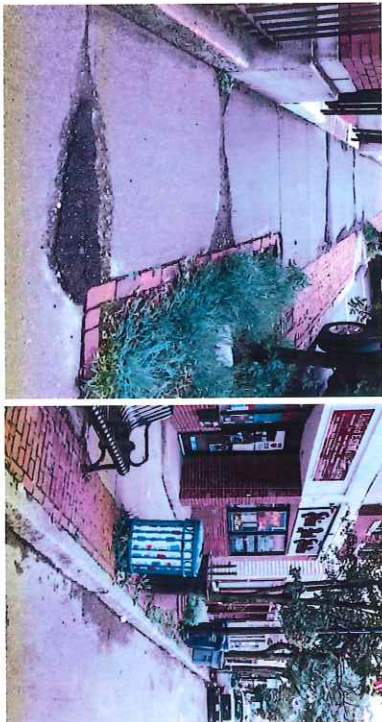
Example of poor sidewalk conditions along Cambridge St.
